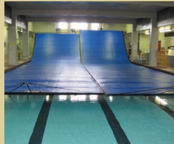
South Park Middle School swimming pool with vapor tight pool cover and energy efficient lighting
