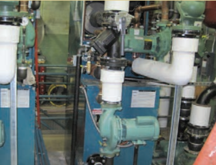
Newly installed water boilers at Emmeline Cook Elementary School
