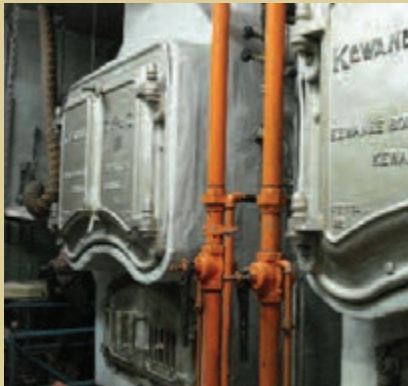
Old steam boilers, which were replaced
